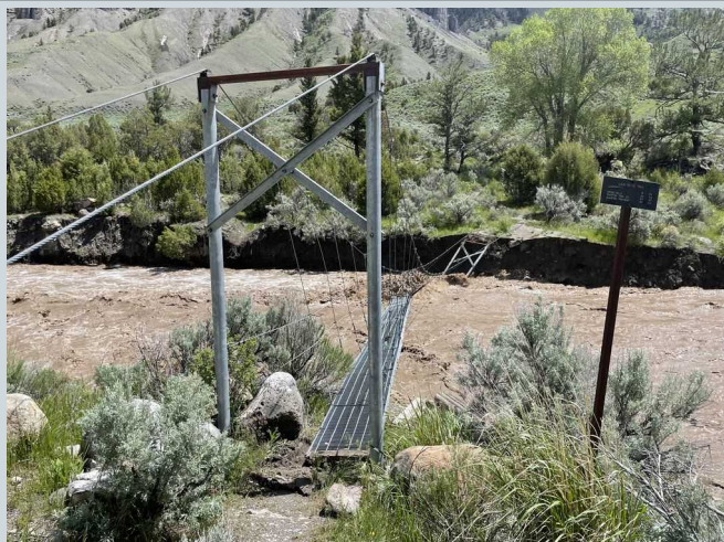
Trail bridge collapsed by flooded Gardiner River
